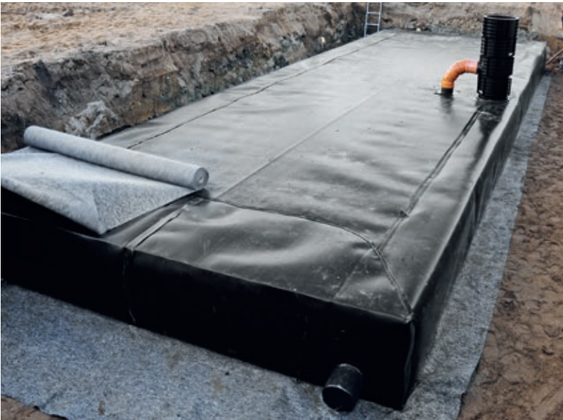
The outer protective fleece is applied once the sealing membrane is complete
