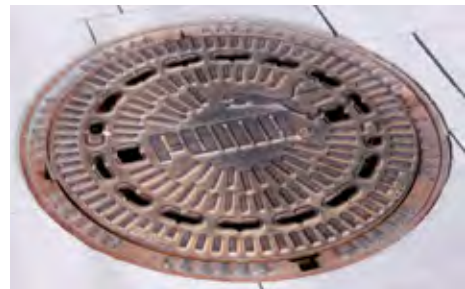
Manhole cover with company logo
