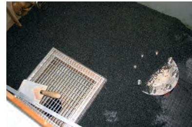
Test set-up with drainage mat and gravel bed in front of the gully top
