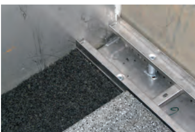
Channel system loosely installed
